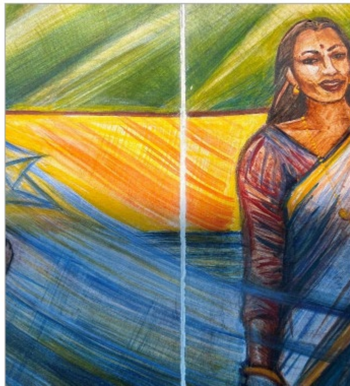
Same area after application of the custom-made mortar and the acrylic filler compound
