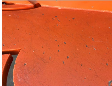
Image 5: Detail view of the orange bench showing repeated impact damage with chips, scratching, and corrosion present.
