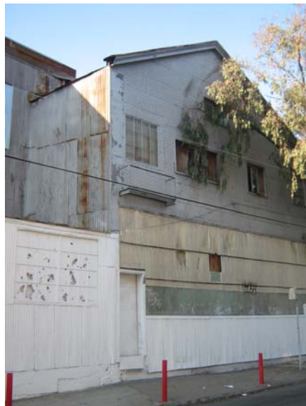
East façade of 160 Kissling Street (far north portion of building). Source: Page and Turnbull
