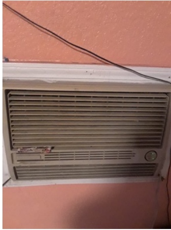
Old, inefficient window ACs
