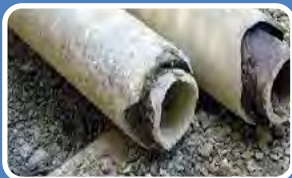
Transite Pipe – Asbestos Containing Material
