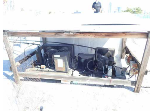
2950-2978 16th St- tenant owned refrigeration condenser unit
