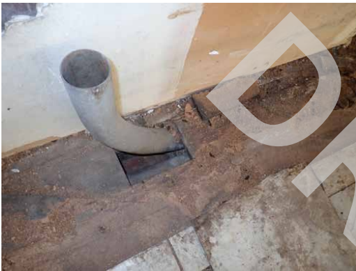
1979 Mission St- dry-rot floor area
