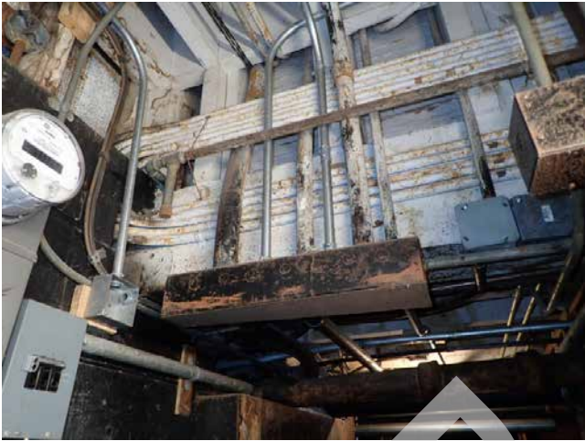
197. 1985 Mission St / 2950-2978 16th St Electrical conduit bundle
