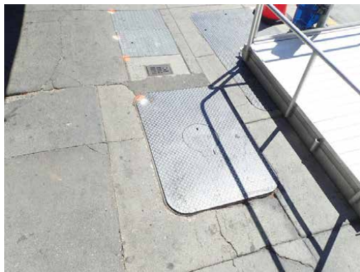
Underground mounted transformer
