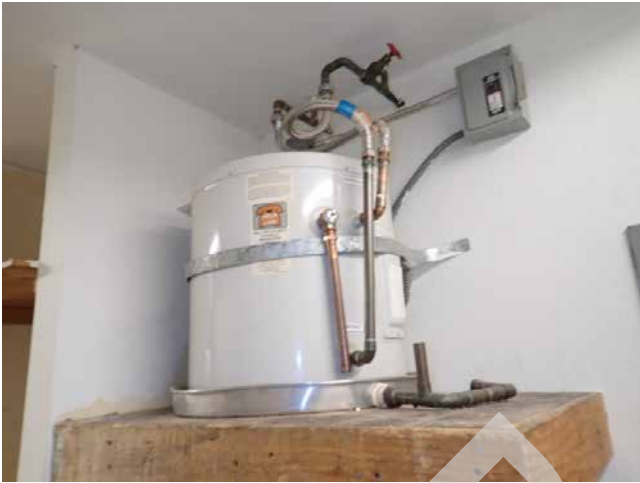
177. Unit 1979 water heater
