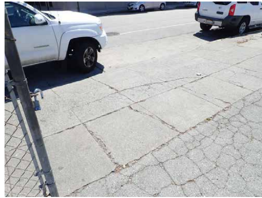
Cracked concrete apron
