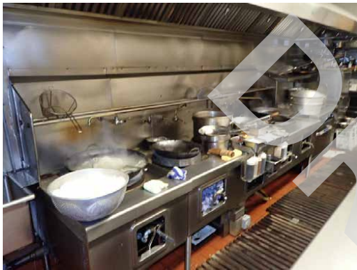
Unit 2960 commercial kitchen
