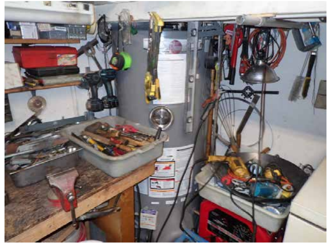
178. Unit 1960 water heater
