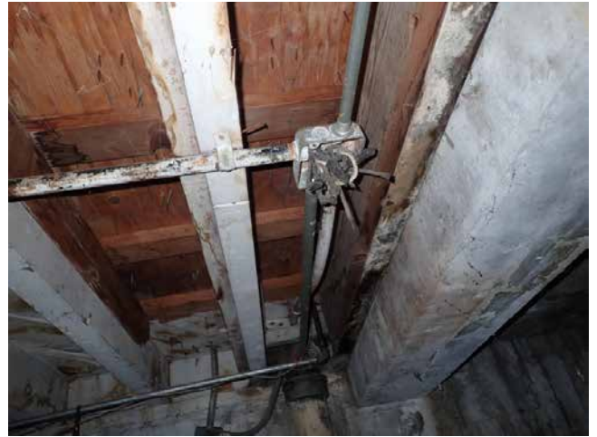
198. 1985 Mission St / 2950-2978 16th St Exposed wires
