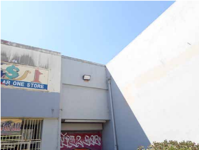
63. Typical building mounted lighting
