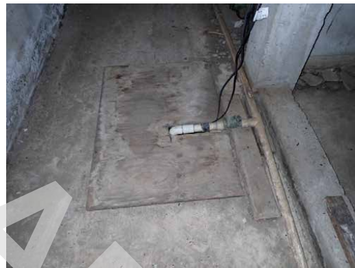
1985 Mission St / 2950-2978 16th St foundationsump pump
