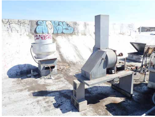
2950-2978 16th St- tenant owned fan equipment
