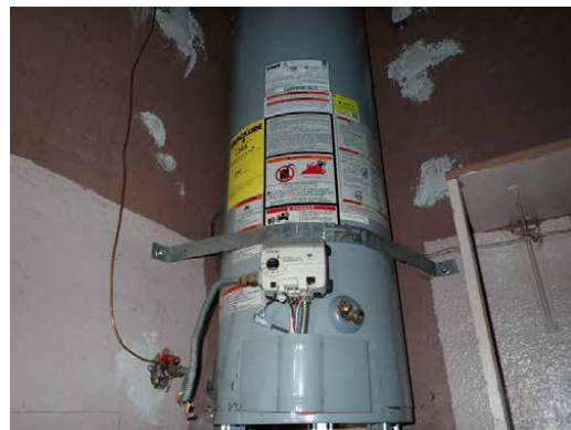
Typical gas water heater
