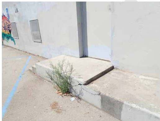
Damage concrete steps
