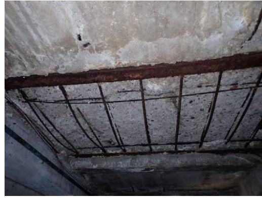
1985 Mission St / 2950-2978 16th St foundation damage to concrete ceiling area
