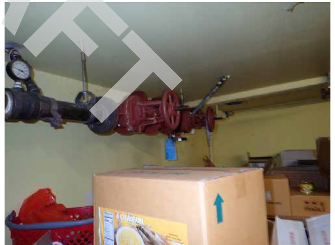
200. 2970 16th St- fire sprinkler backflow device
