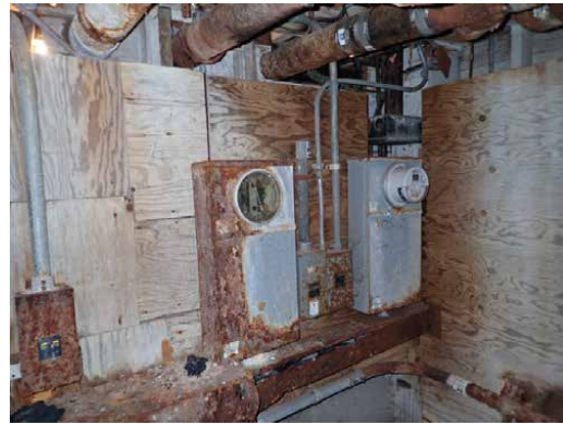
1985 Mission St / 2950-2978 16th St- rusty electrical panel
