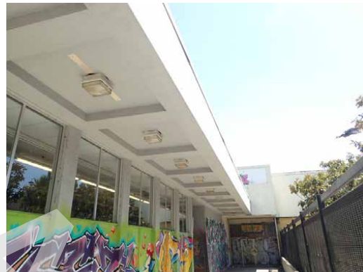
Soffit mounter lighting
