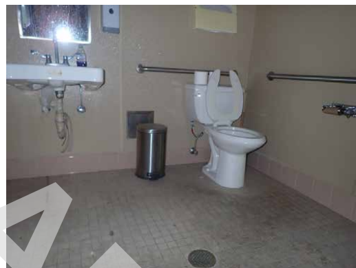
1979 Mission St- piping wrapping is starting to fall off
