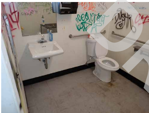
Unit 1985- area under sink not protected
