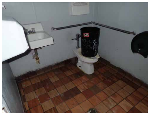
2978 16th St- area under sink not protected
