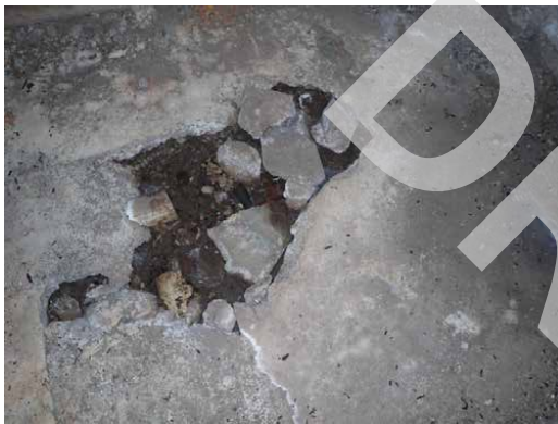
1985 Mission St / 2950-2978 16th St basement area-damaged concrete slab floor
