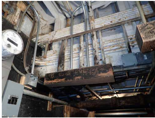
1985 Mission St / 2950-2978 16th St Electrical conduit bundle
