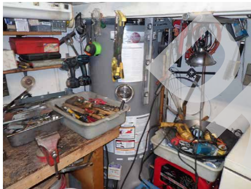
Unit 1960 water heater missing seismic straps
