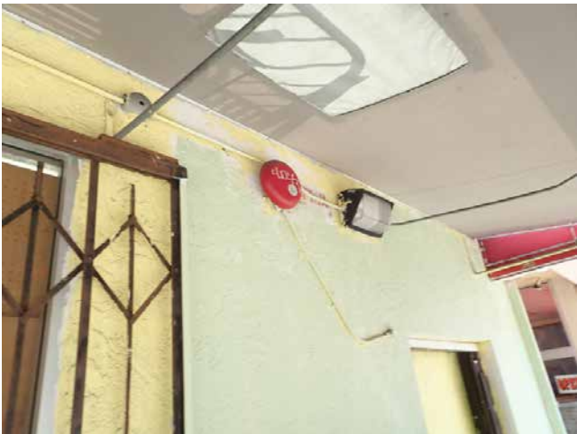
199. 2970 16th St- fire alarm bell
