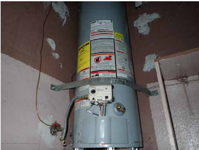
179. Unit 1950 water heater
