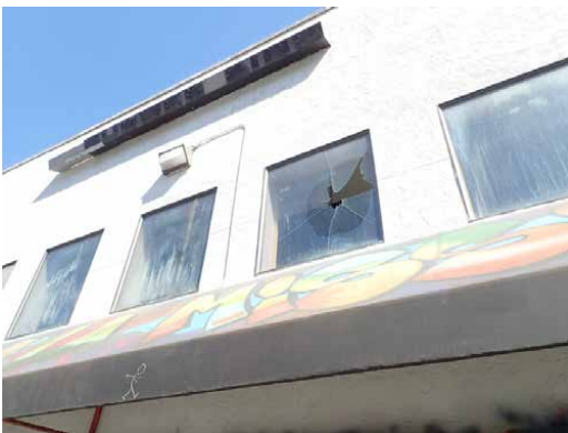
2978 16th St- broken window
