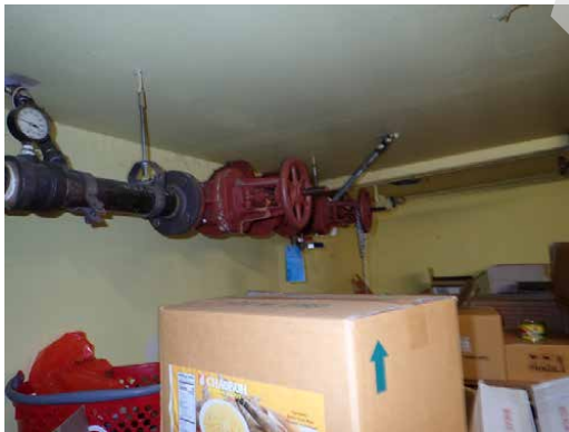
2970 16th St- fire sprinkler backflow device
