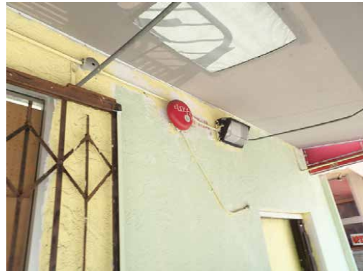
2970 16th St- fire alarm bell
