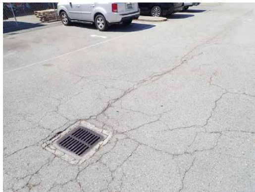
Typical asphalt cracking
