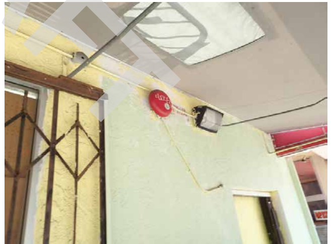
60. Fire alarm bell for 2970-2972 16th St.
