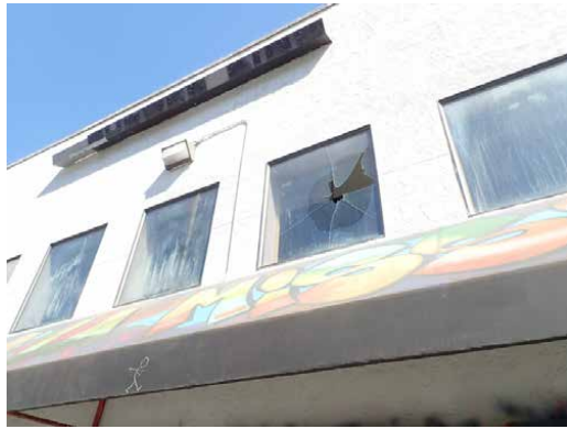
2978 16th St- broken windows
