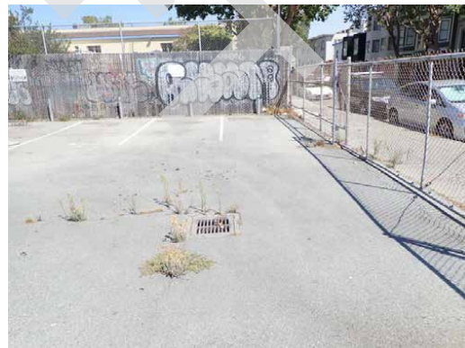
Weeds in asphalt cracks
