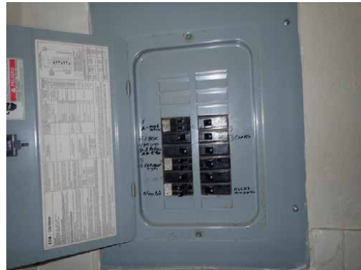
Typical electrical panel
