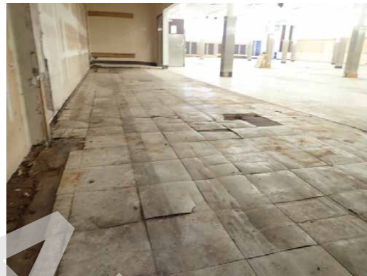
1979 Mission St- dry-rot floor area
