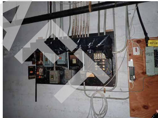
1985 Mission St / 2950-2978 16th St- old electrical equipment
