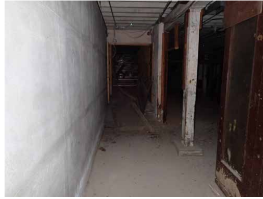
1985 Mission St / 2950-2978 16th St wood column support in basement area
