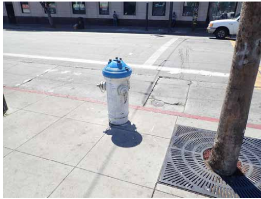
Typical fire hydrant
