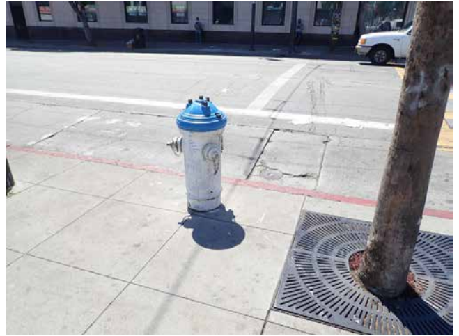
202. Typical fire hydrant
