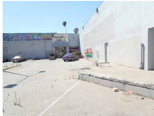
Loading dock area with damaged concrete- 1979 Mission St
