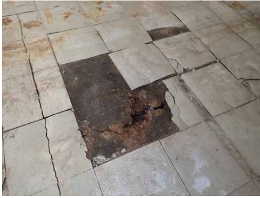
1979 Mission St- appears to be dry-rot damaged to wood flooring
