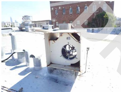
2950-2978 16th St- tenant owned fan unit
