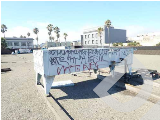
1979 Mission St- condenser unit
