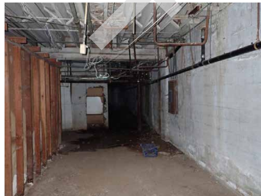
Basement Area-concrete slab foundation with concrete sidewalls at 1985 Mission St / 2950-2978 16th St
