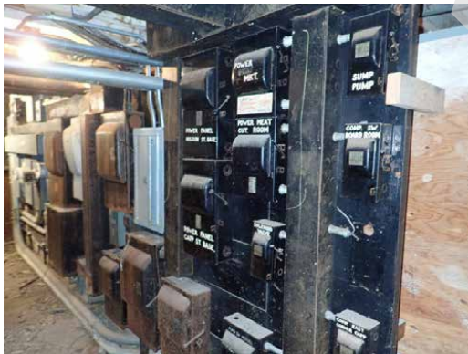
1985 Mission St / 2950-2978 16th St- old electrical switch equipment
