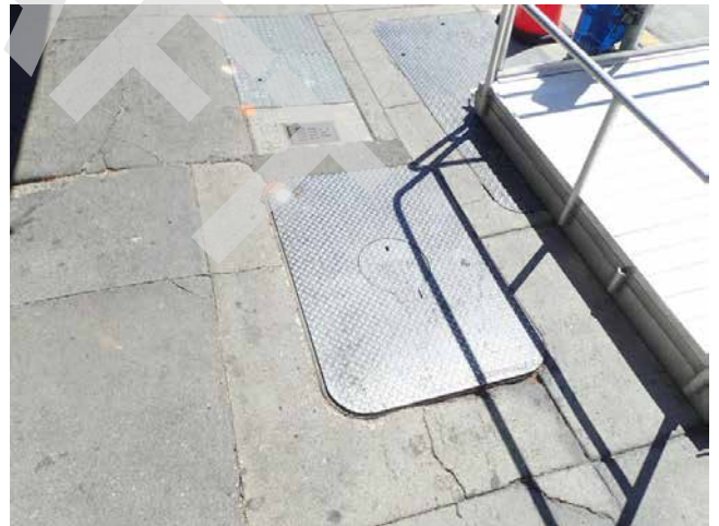
48. Underground mounted transformer
