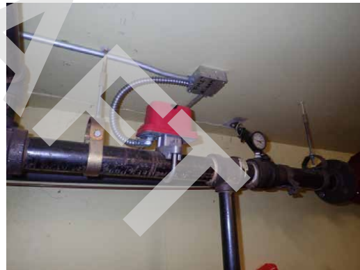
2970 16th St- fire riser pipe
