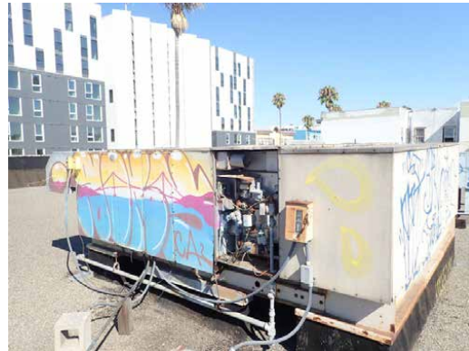
1979 Mission St- air handler with furnace
