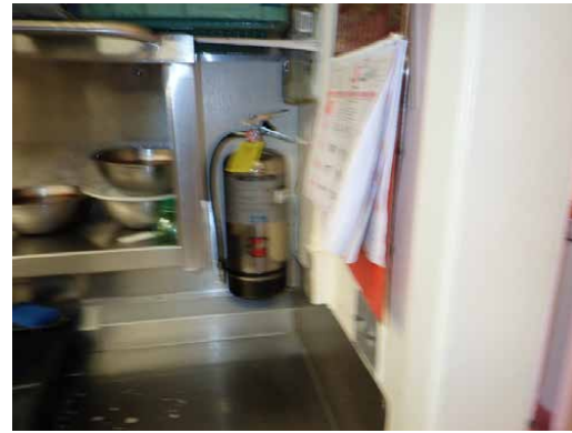
2960 16th St- fire extinguisher
