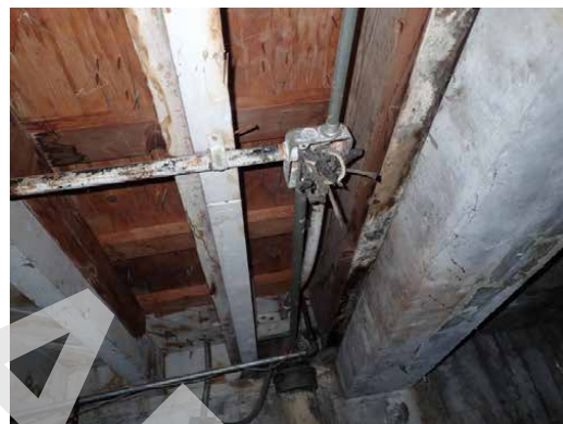
1985 Mission St / 2950-2978 16th St Exposed wires
