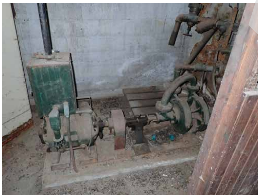
Unit 1985- abandoned hydraulic lift
