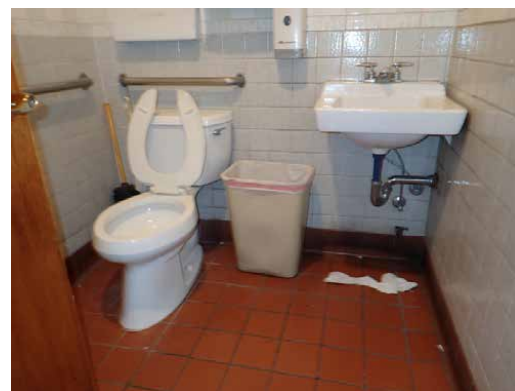
2960 16th St- area under sink not protected
