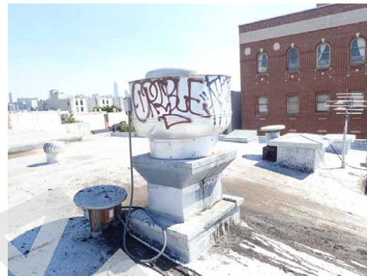
2950-2978 16th St- tenant owner cooking hood fan
