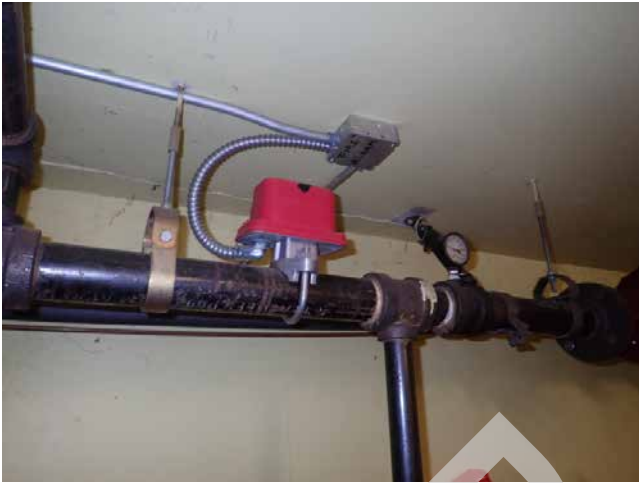
201. 2970 16th St- fire riser pipe
