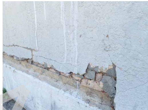
Damaged stucco over wood north side of 1985 Mission St.
