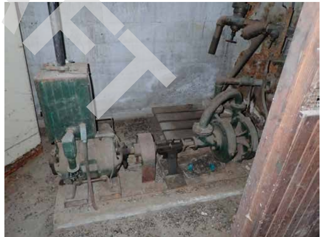
276. Abandoned hydraulic lift
