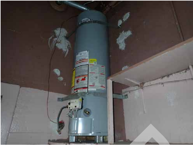
181. Unit 1950 water heater
