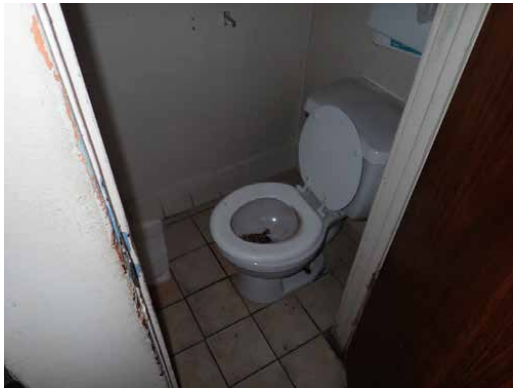
2950 16th St- restroom toilet area not ADA compliant
