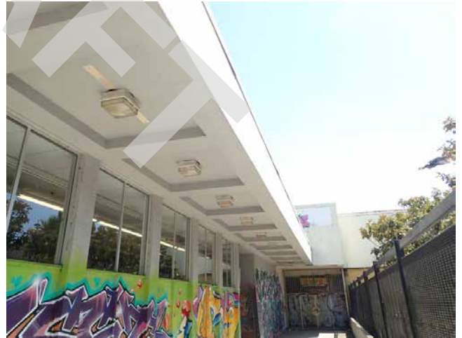
64. Soffit mounter lighting
