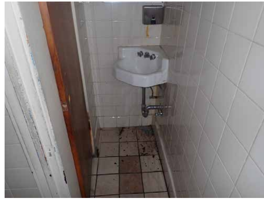
2950 16th St- clearance area around sink not ADA compliant
