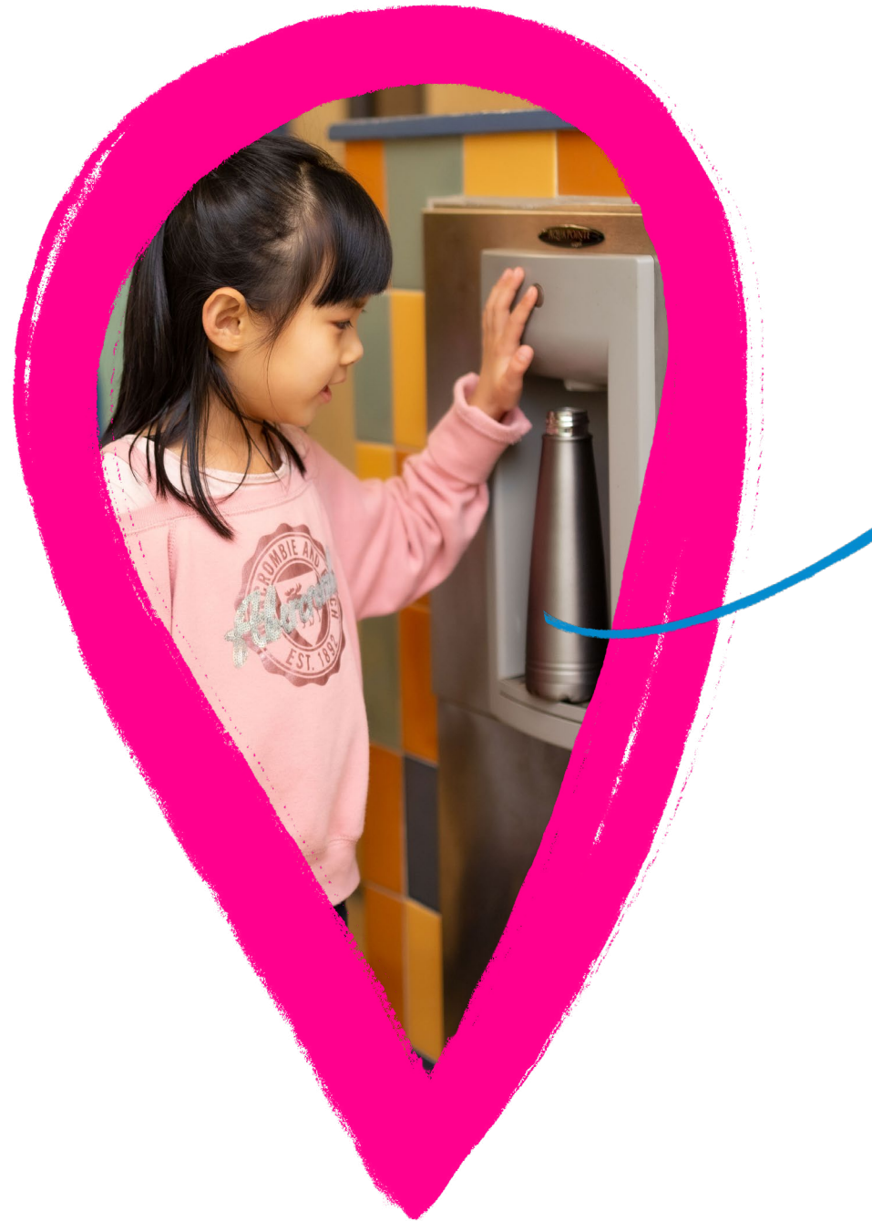
Water bottle filling station at school
