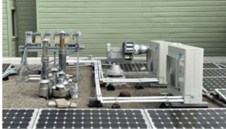
New Mechanical Ductwork and Equipment
