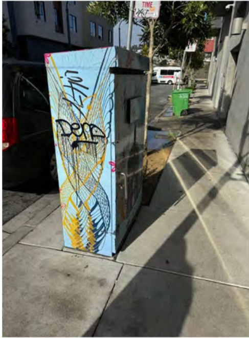
3. On Lee, at Ocean, northeast corner, outside 1140 Ocean, 1 box
