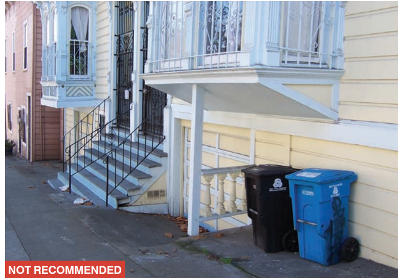
The base of this historic projecting bay was adversely impacted for this garage. This treatment does not meet the criteria for inserting a garage within an existing structure.
