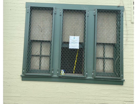
MANY WINDOWS BROKEN AND BOARDED UP
