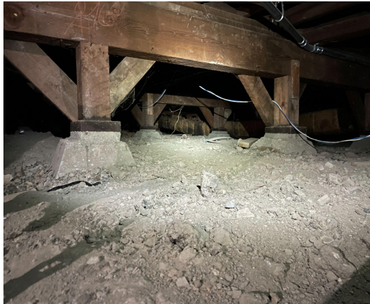
FOUNDATION REQUIRES UPGRADES
