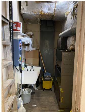
MEP SYSTEMS INEFFICIENT
