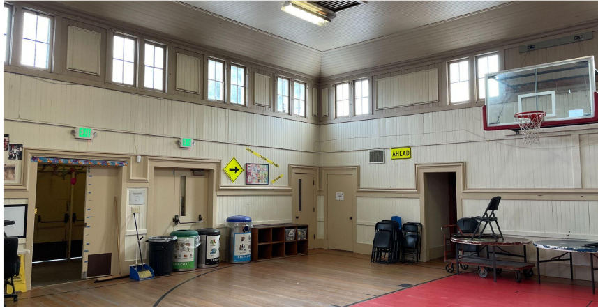
CLUBHOUSE HAS SIGNIFICANT SETTLEMENT, SEISMIC UPGRADE REQ'D
