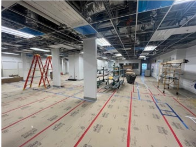
Primary Core Lab (Automation Line)
