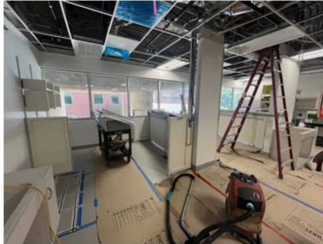
Testing and Workstation Space
