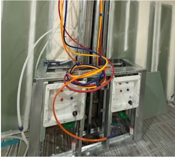
Dialysis Equipment Piping/Tubing
