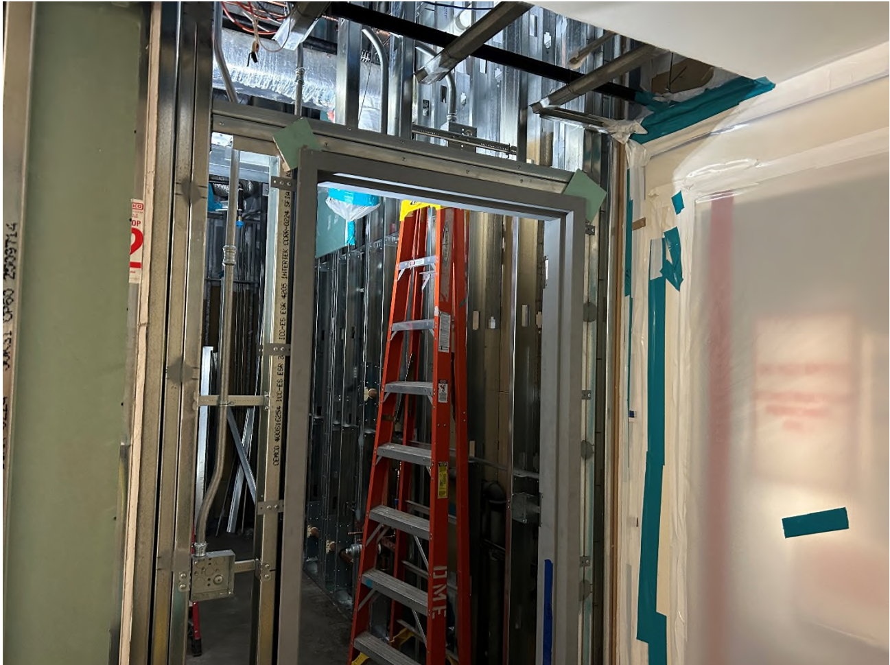
Door frame, metal stud, and electrical conduit installation at Shower Room GL-8
