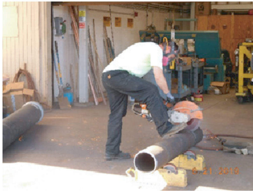
Fabrication Shop workers cut pipe at exterior of shop. Hazardous debris is not contained.
