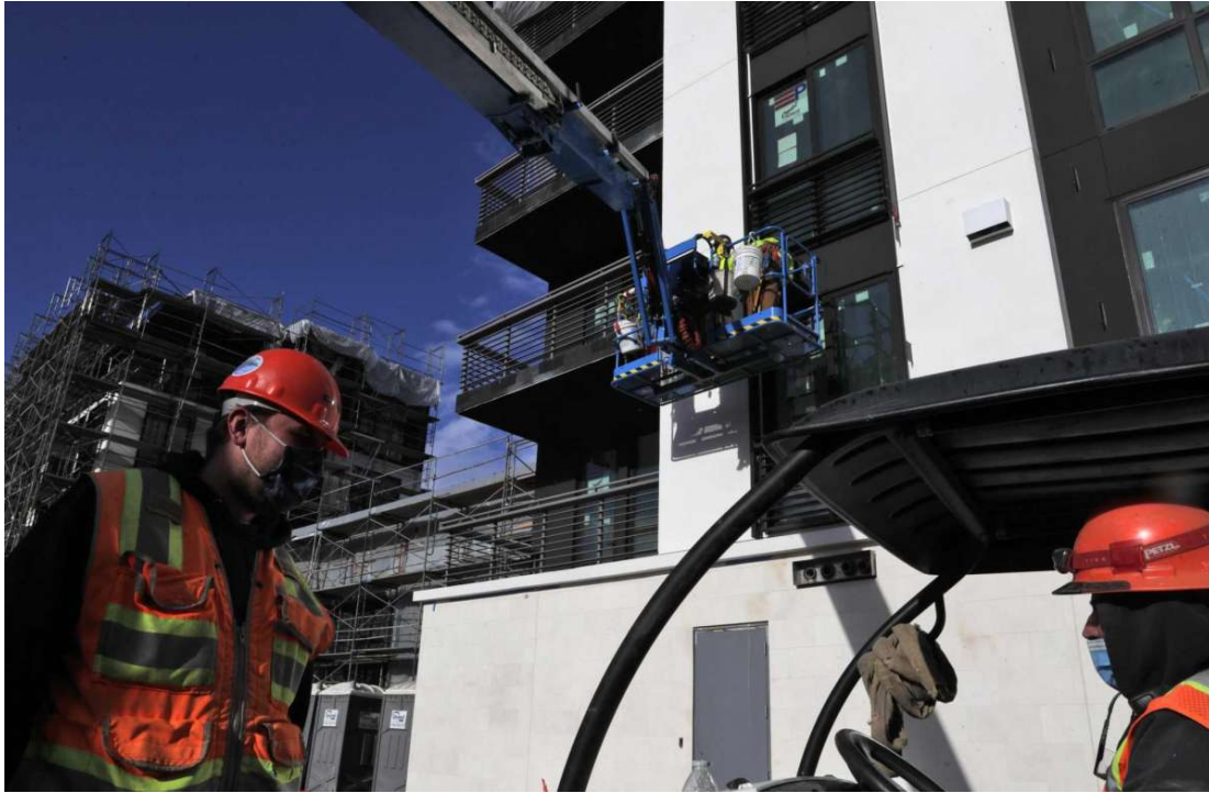
Construction continues on the new Bristol Condominiums on Yerba Buena Island in San Francisco.
